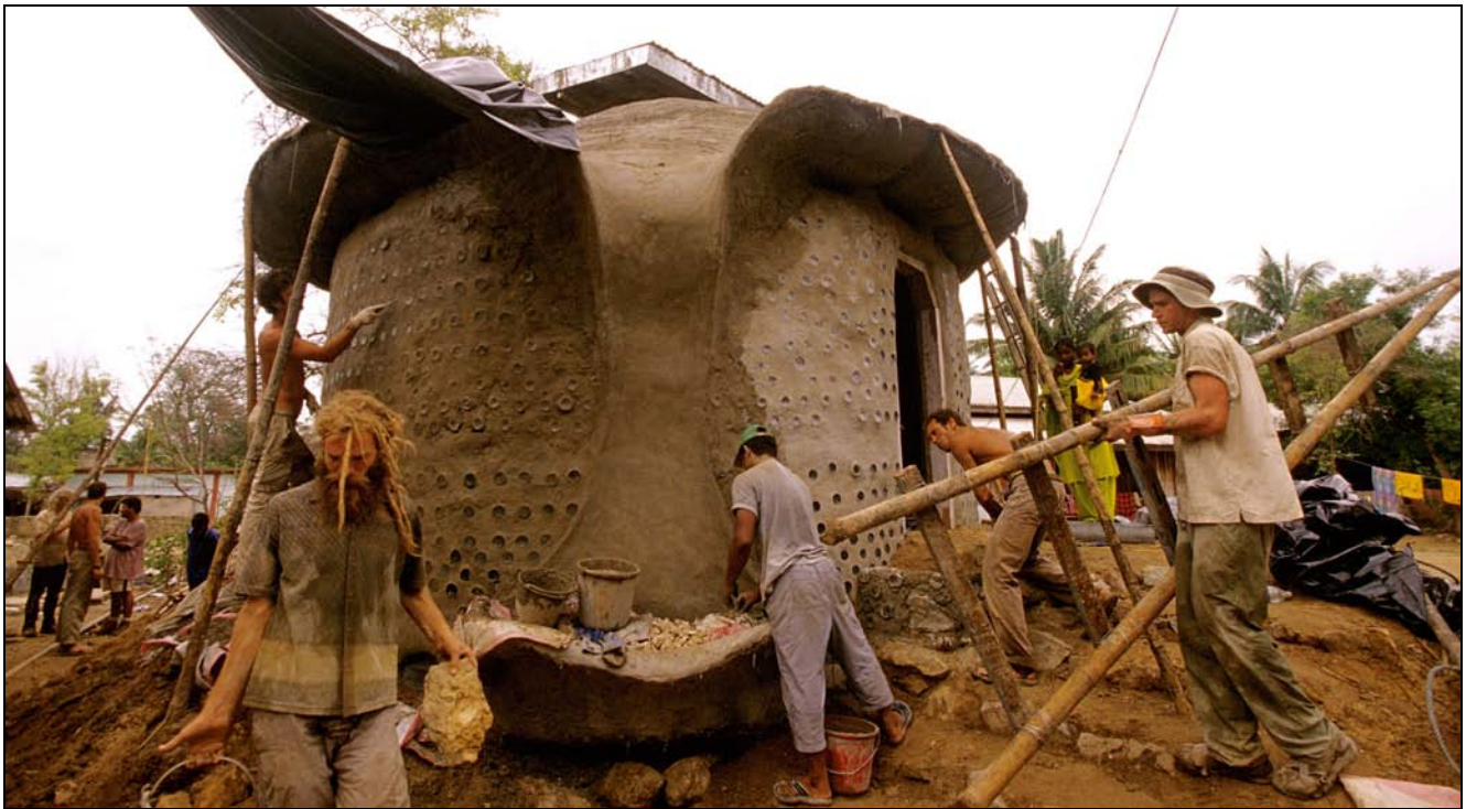
Reynolds' crew at work in India with the Andaman Islands tsunami relief project.
